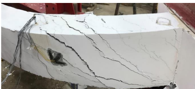
Fig. 9 Specimen C3 failure.
